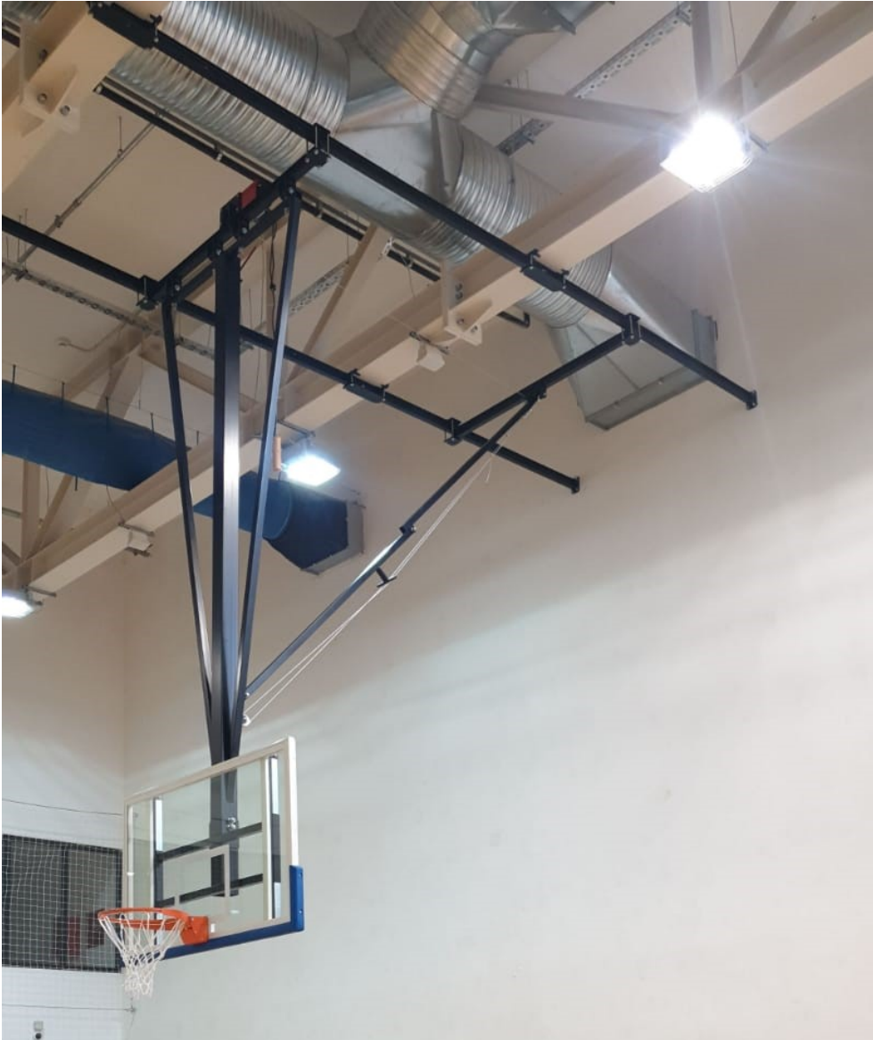
Roof mobile basket system, wood backboard.
